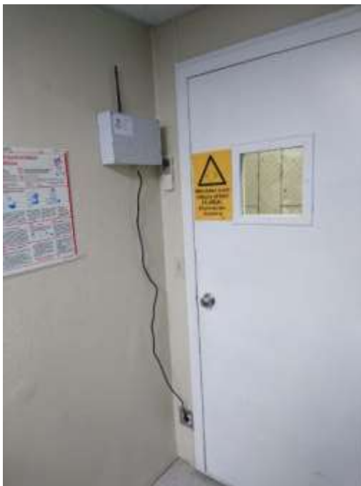
Lora Access Point at the wall in the control room
